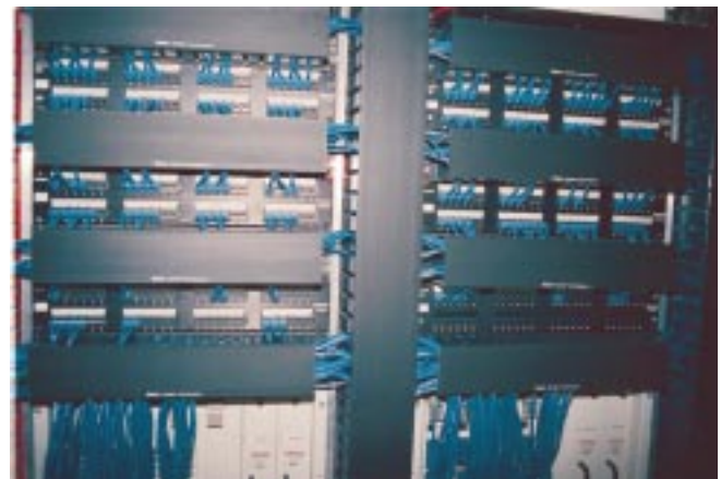
Data-electronic racks maintain a blown-fiber infrastructure in which fiber will be blown from the intermediate crossconnect and terminated at each work area.
