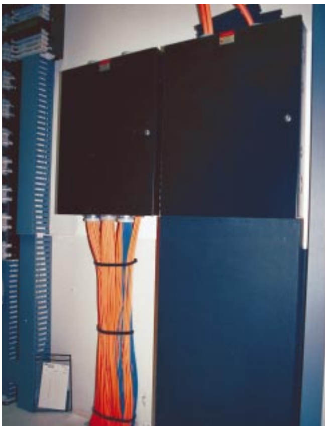
Routed to the 18 intermediate crossconnects throughout the facility, empty Microduct tubes are capped and labeled, ready to receive optical fibers whenever needed.
