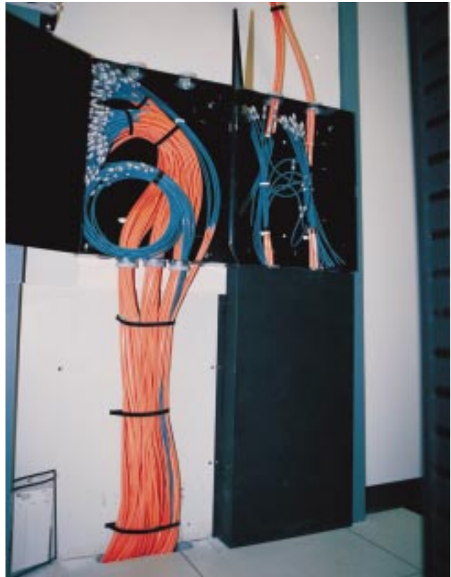
Ready for future installation of blown optical fibers, Multiduct cables containing individual tubes are consolidated in wall boxes at the intermediate crossconnect.
